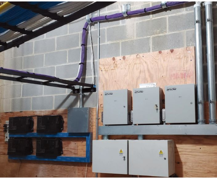
Above: One of six IDF/MDF closets in the Consortium contain components that support the facility's access, camera, and paging solutions, including Honeywell access control panels, Altronix power supply enclosures, and low-voltage structured cabling.
