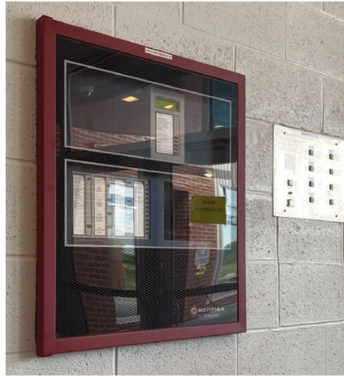
Right: In case of emergency, Advantech integrated a Honeywell Notifier fire alarm system and bi-directional amplification system. For quick communication and correspondence, panic/lockdown buttons and a Bogen public address system were included.
